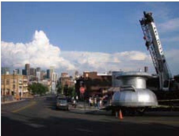
Top: 4- by-8-foot metal sheets were welded, then temporarily strapped to the steel substrate to avoid oil-canning. Contractor Tom Hewitson of Miramar Construction developed a gauge or template to maintain the desired circumference as the steel was erected.
